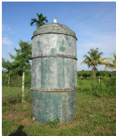
Figure 11. Plant in B1, bio-digester
