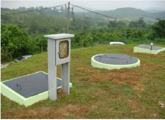
Figure 1. Plant in C1, bio-digester
