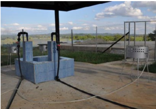
Figure 3. Plant in C3, bio-digester
