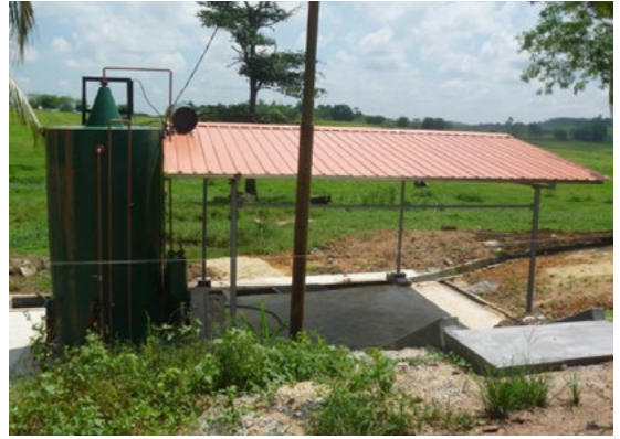
Figure 2. Plant in C2, bio-digester
