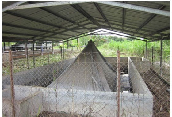
Figure 4. Plant in C4, bio-digester
