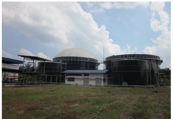
Figure 10. Plant in P3, bio-digester
